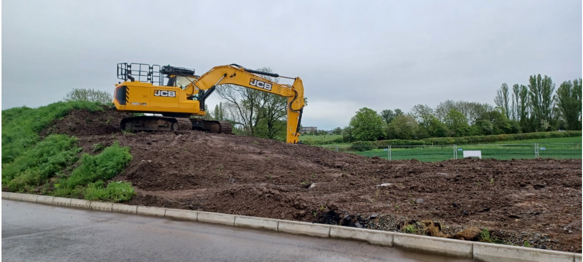
Figure 5 - Incomplete earth bund along southern site boundary
